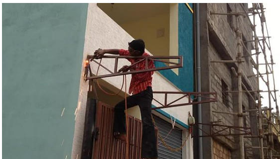
Man welding a metal structure in a newly constructed house in Bengaluru, India
